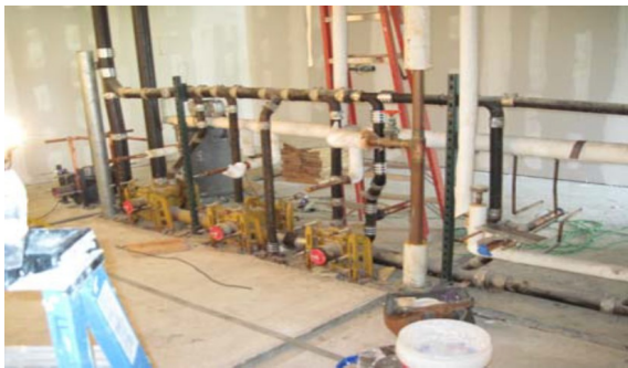
Plumbing in restroom batteries
